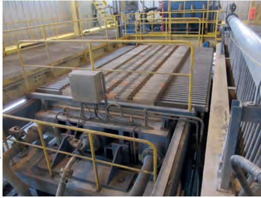
Left: Tailings filtration equipment allows the Marlin mine to efficiently reclaim process water
